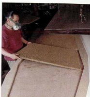
Work from the bottom up. After applying glue to the bottom skin, place the MDF frame and the honeycomb material in place. Fasten the frame to the skin with screws.
